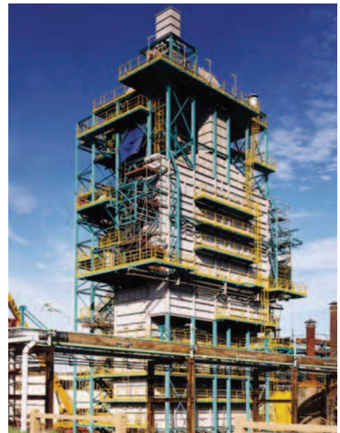
Ethylene Cracker Unit
