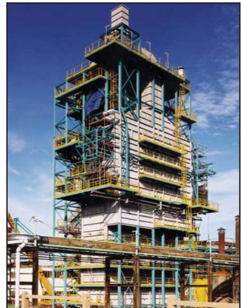
Ethylene Cracker Unit
